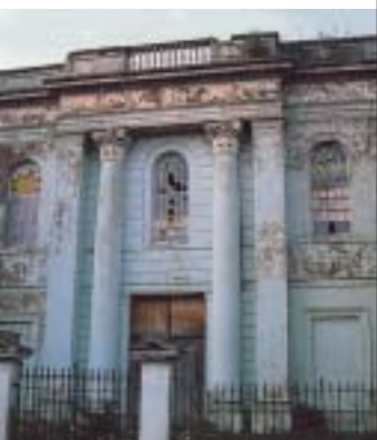
Above: Glendower Street Chapel in derelict state (Anthony Jones).
